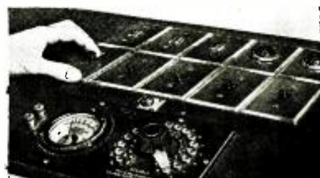
Fig. D The switching panel at the American Foundation for the Blind, for turning on the beams between different offices and rooms. An operator turns on the desired beams as needed.
